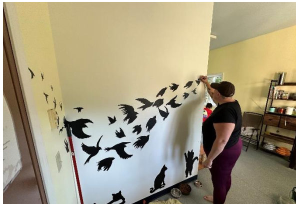
Renovations of the adult cat room with grant funding from the Alaska Community Foundation, November 2023.
